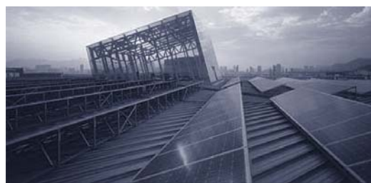
Fig. 2 Solar panels on the roof of the EMSD Headquarters
